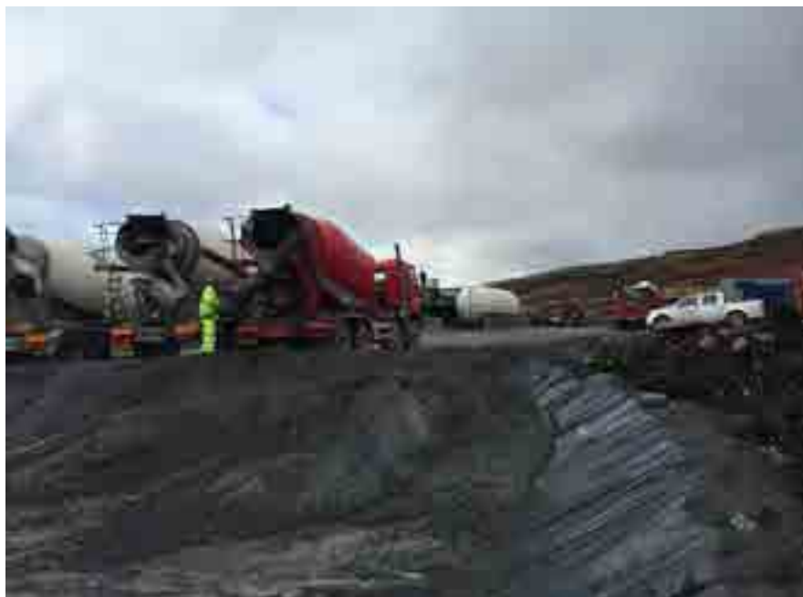
Plate 10: Typical concrete wash-out facility
