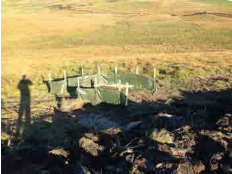
Plate 1: Typical silt fencing
