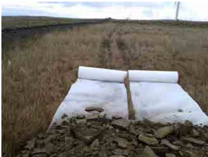
Plate 13: Semi-permeable geotextile layer
