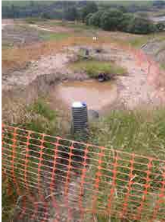
Plate 5: Typical lagoon and flocculent station
